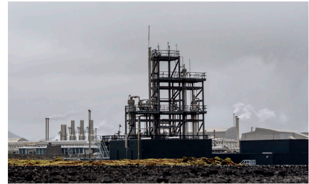
Renewable methanol plant in Iceland. Source: Carbon Recycling International
